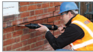
3. Using the Helifix Pointing Gun, inject a bead of HeliBond along the back of the slot
