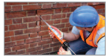
6. Re-point the mortar bed and make good the vertical crack with CrackBond TE
