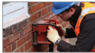
1. Rake out or cut slots into the horizontal mortar beds, a minimum of 500mm either side of the crack
